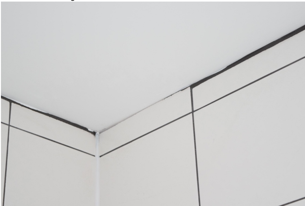
Shower room ceiling sealant not consistent all around
