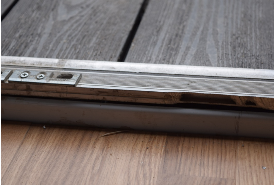
Upstairs French door cill not right & daylight showing under
