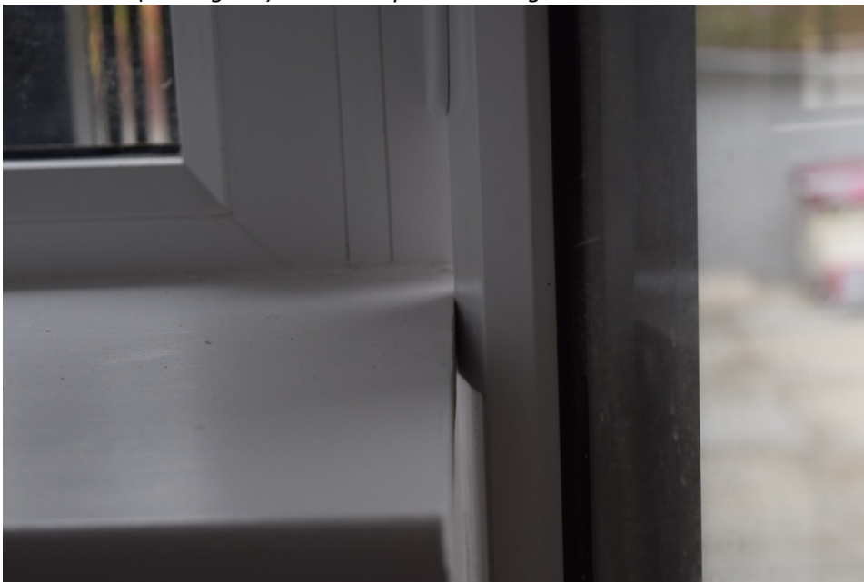
Door on LHS (looking out) does not open to 90 degrees due to window cill
